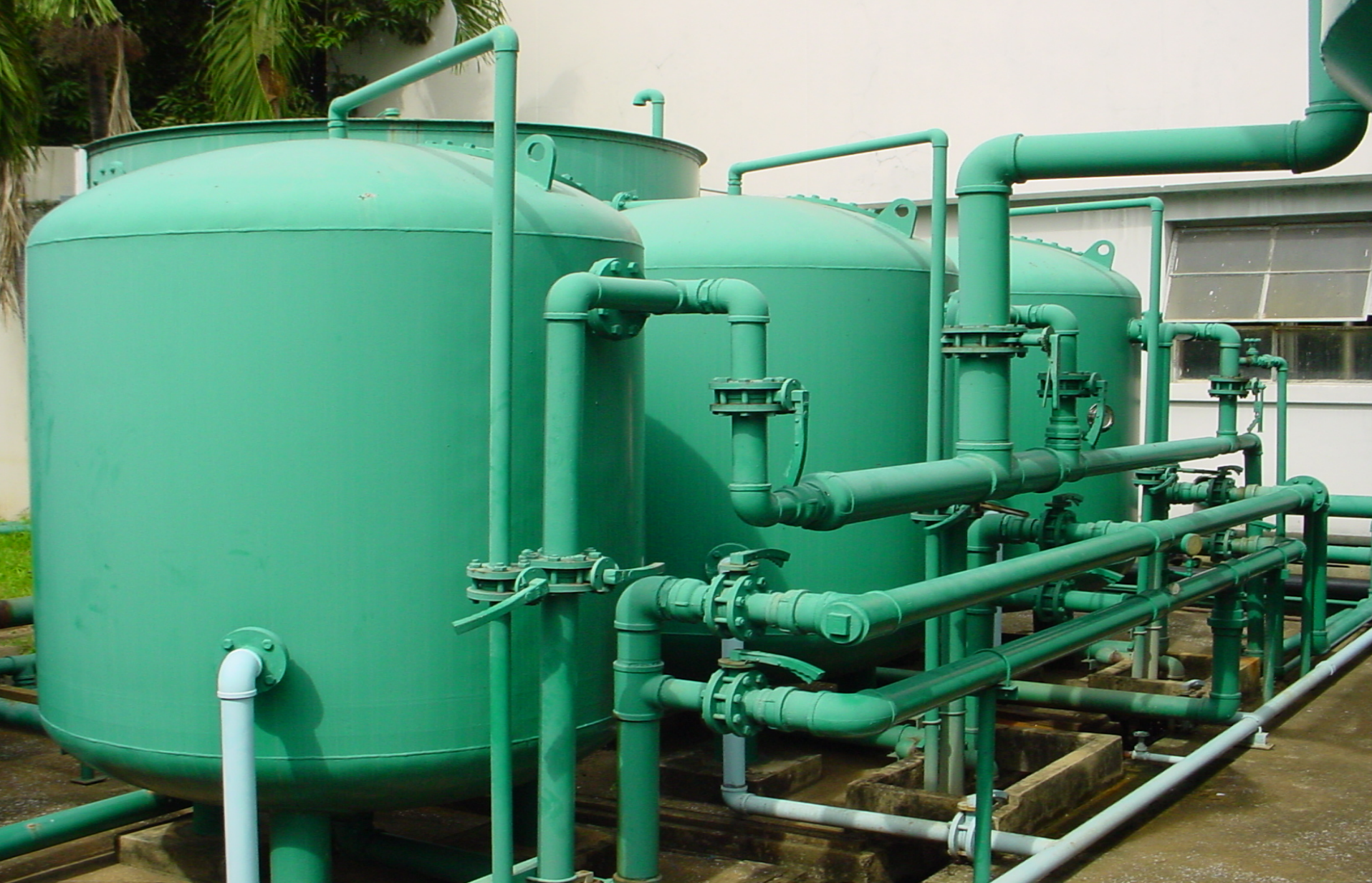
Vertical Pressure sand filter
