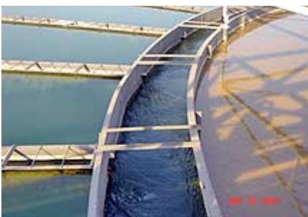
Water from the Chao Phraya River flows through a clarifier and a filter at the Bangkhen water treatment plant.
