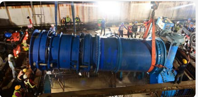
Condition assessment and rehabilitation of water transmission tunnel along Prasert-Manukitch Road, and tunnel interconnection works at Min Buri Pumping Station
